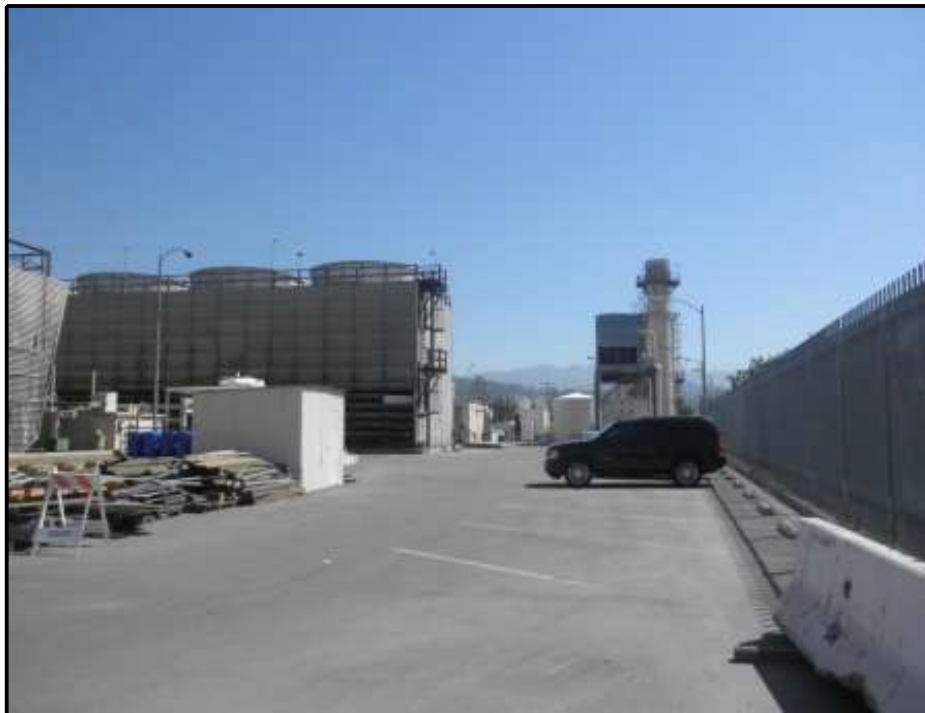
Figure 19. Cooling Tower No. 1 (Generator No. 9 in Background), View Looking East (Photo by J. Terry).
