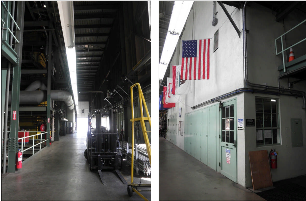
Figure 29 Grayson Boiler Building: Overview of First Floor, View Looking North (left); Control Room, View Looking Southwest (right)
