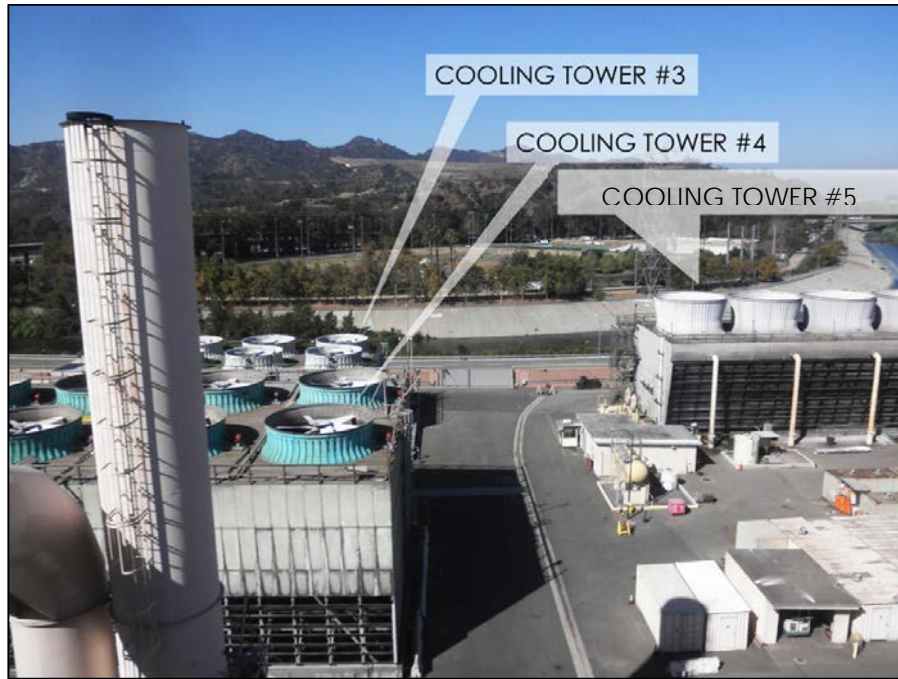
Figure 5 Overview of Project Area from Roof of Grayson Boiler Building Looking West
