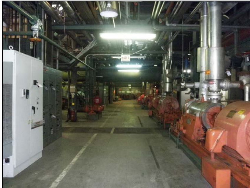
Figure 27 Grayson Boiler Building: Interior Overview of Basement Floor Level, View Looking North
