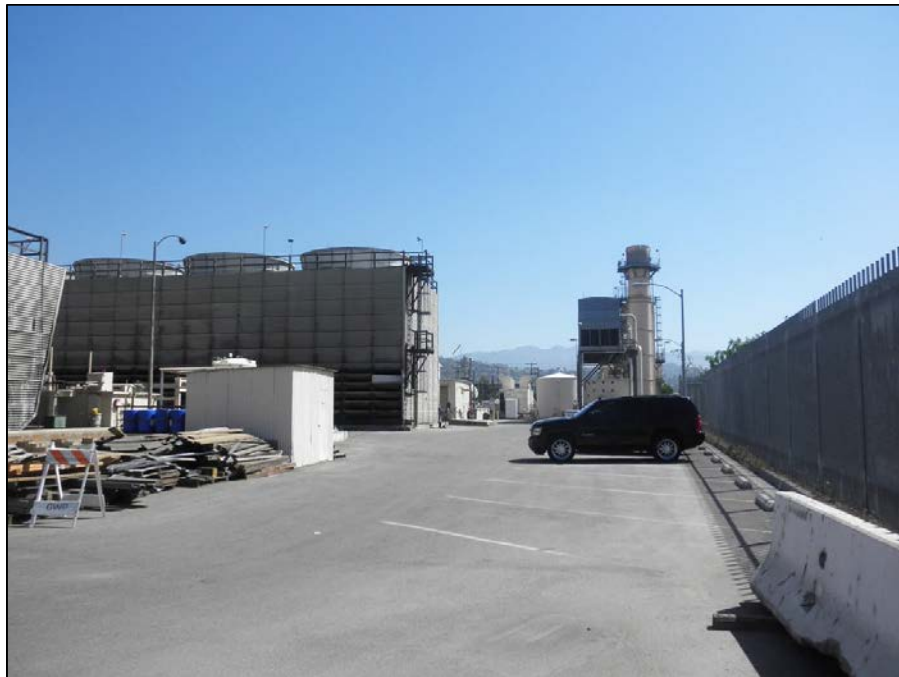
Figure 37 Cooling Tower No. 1 (Generator No. 9 in Background), View Looking East
