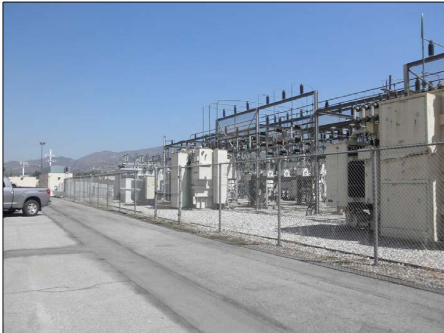
Figure 42 Kellogg Switching Station, View Looking Northeast
