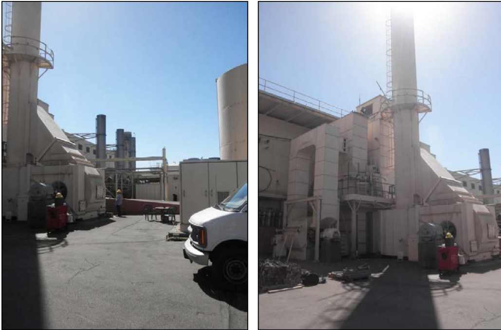
Figure 25 Grayson Boiler Building: Southwest Elevation Looking at Boiler Stacks for Boilers 1 and 2 Center Rear as well as Boiler 3 in far left (right), Boiler 3 (right). View Looking Southeast
