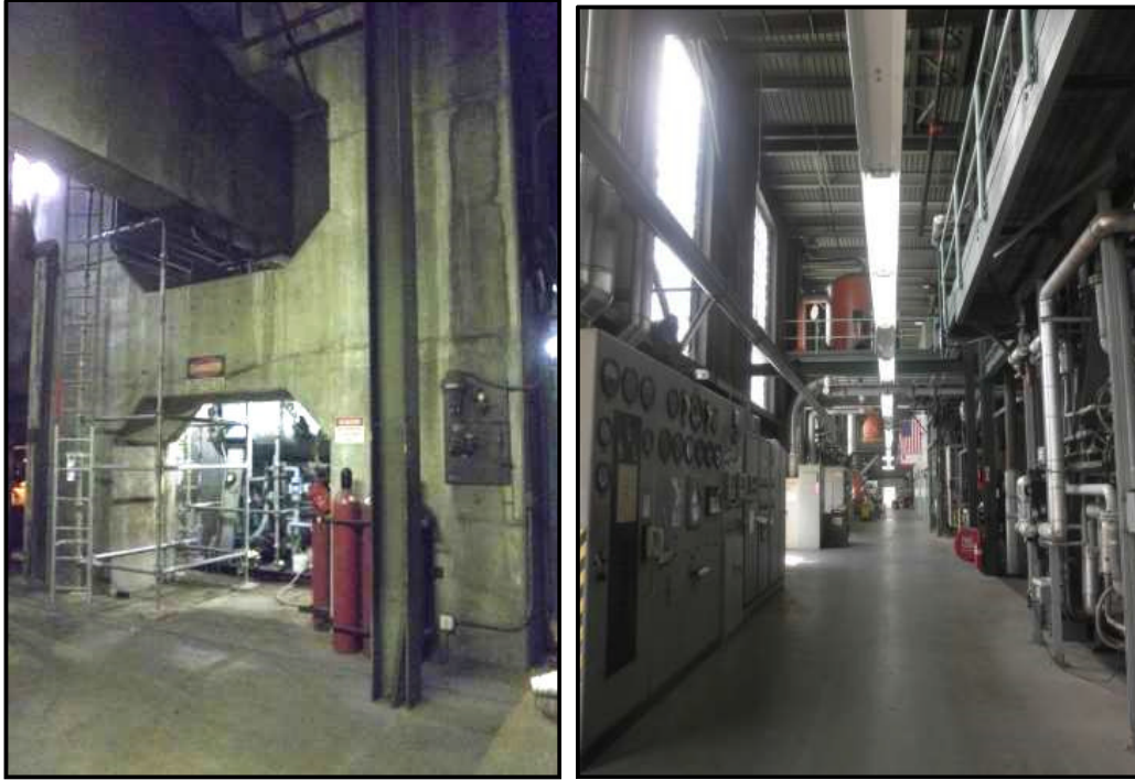
Figure 13. Basement Level Depicting Concrete Structure below Turbine and Generator 1, View Looking Northeast (left); Overview of Main Level, View Looking South (right). (Photo by J. Terry).
