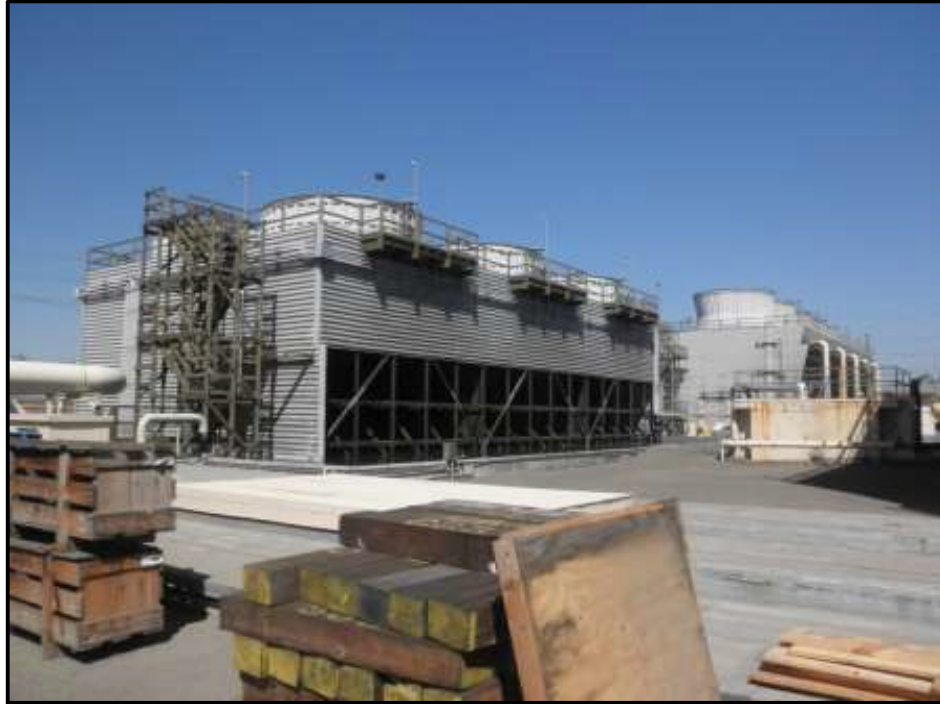
Figure 21. Cooling Tower No. 3 (Cooling Tower No. 5 in Background), View Looking Northwest (Photo by J. Terry).
