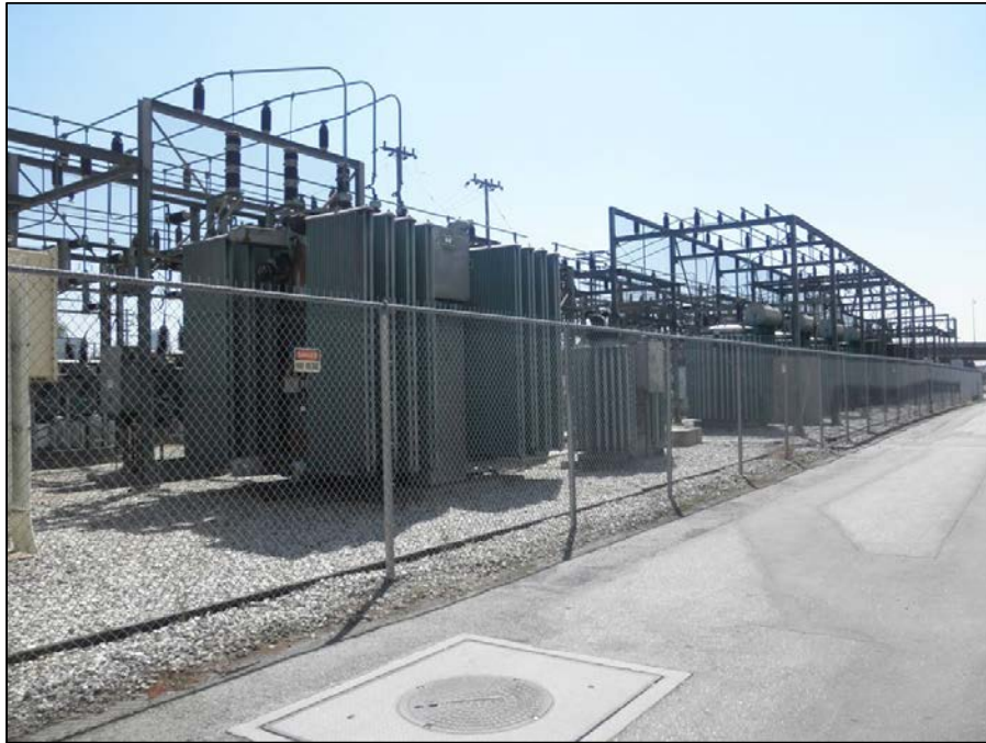
Figure 43 Glendale Switching Station, View Looking Southeast
