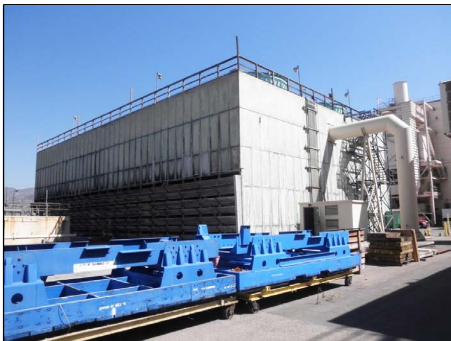
Figure 40 Cooling Tower No. 4, View Looking Northeast
