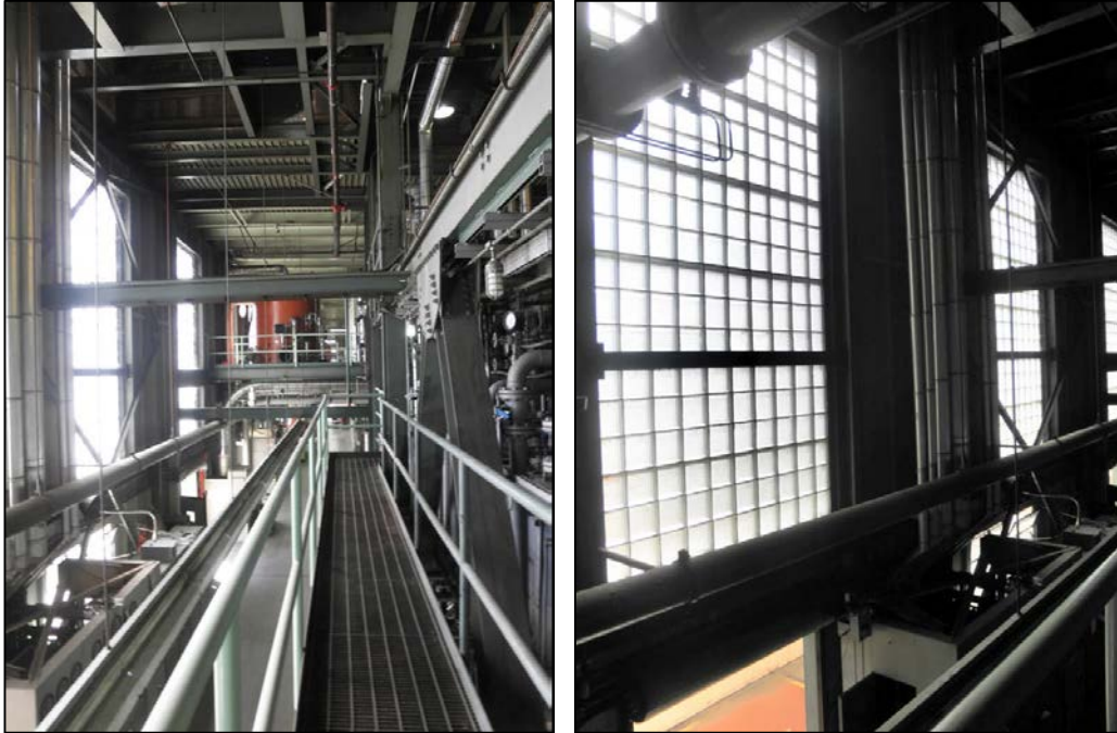
Figure 33 Grayson Boiler Building: Mezzanine, Looking Southeast (left); Structural Glass Block Windows on Northeast Elevation (right), Looking Southeast
