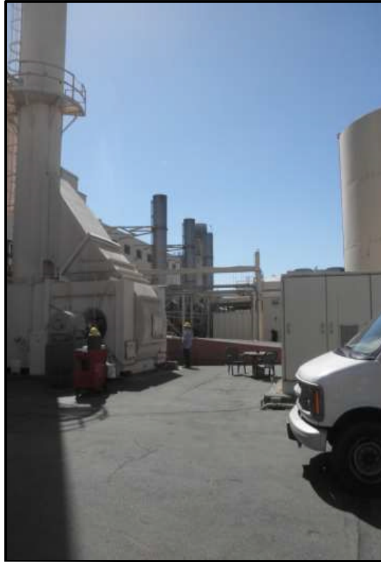
Figure 11. Boiler Stacks (Boilers 1 and 2 Center Rear of Photograph; Boiler 3 to Left), View Looking South. (Photo by J. Terry).
