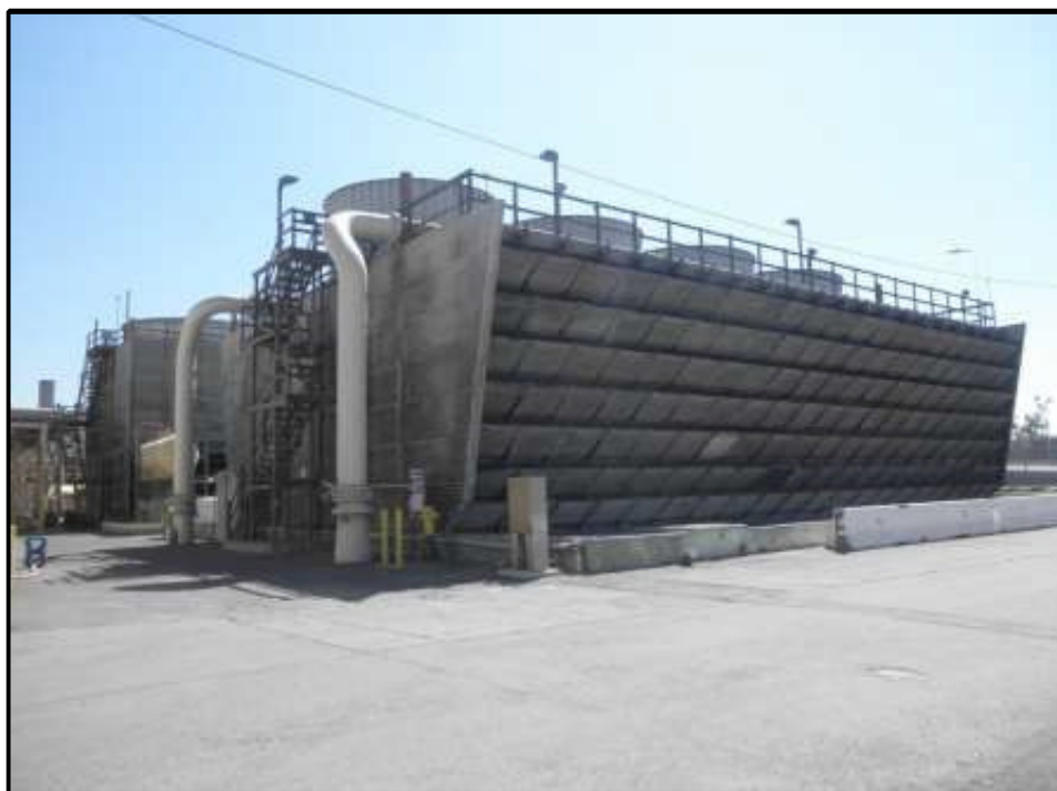
Figure 20. Cooling Tower No. 2 (Cooling Tower No. 1 in Background), View Looking Southeast (Photo by J. Terry).
