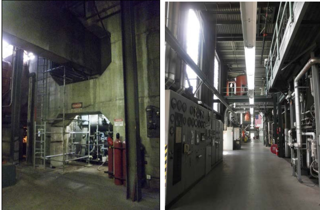
Figure 28 Grayson Boiler Building: Basement Level Depicting Concrete Structure Below Turbine and Generator 1, View Looking Northeast (left); Overview of Main Level, View Looking South (right)
