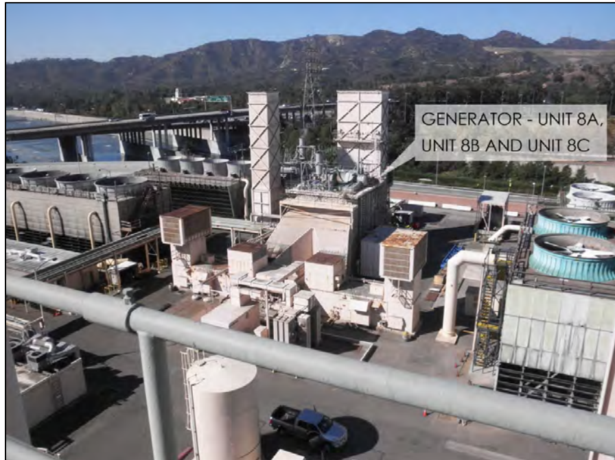
Figure 6 Overview of Project Area from Roof of Grayson Boiler Building Looking Southwest
