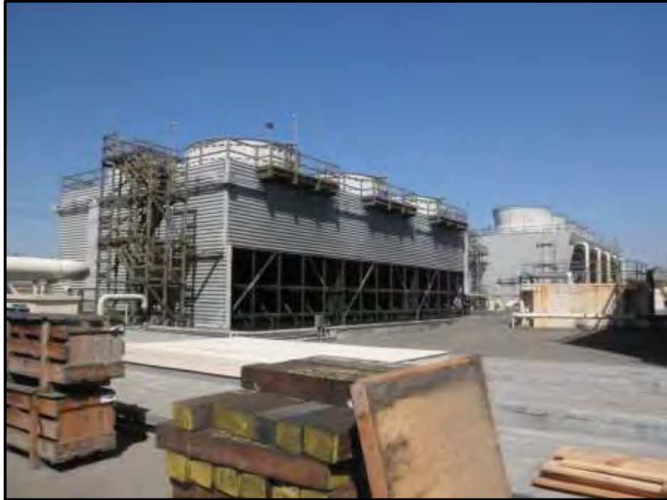
Photograph 13. Cooling Tower No. 3 (No. 5 in Background), View Looking Northwest (Photo by J. Terry).
