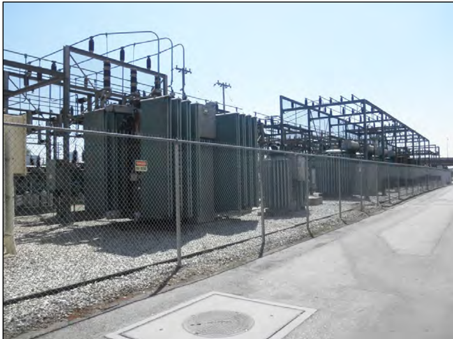
Figure 43 Glendale Switching Station, View Looking Southeast
