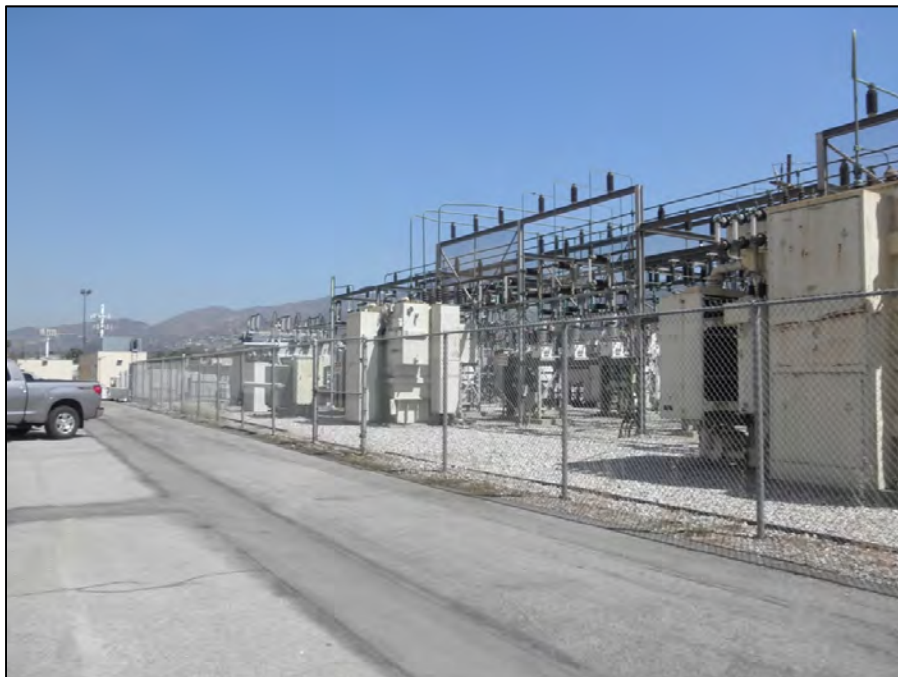
Figure 42 Kellogg Switching Station, View Looking Northeast
