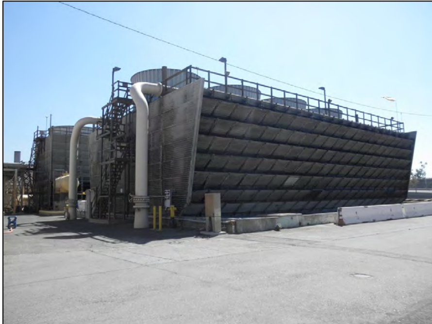
Figure 38 Cooling Tower No. 2 (Cooling Tower No. 1 in Background), View Looking Southeast
