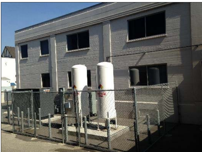
5. View of generator and ASTs with Building A at rear
