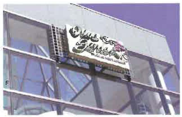
EXISTING OLIVE GARDEN WALL SIGN TO BE REMOVED AND RELOCATED (EXISTING SIGN FRAME & BOX: 10'-6"W x 9' D x 4'-3"H)
