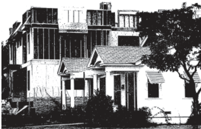
Stalled apartment construction next to single family residences near California Street and Chester Street. Source: "Fight Brewing Over Growth," Los Angeles Times , August 14, 1988.
