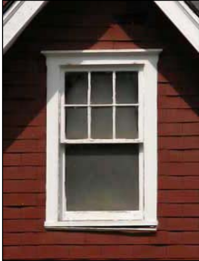
Flat wood window trim is a typical feature of many wood-clad buildings
