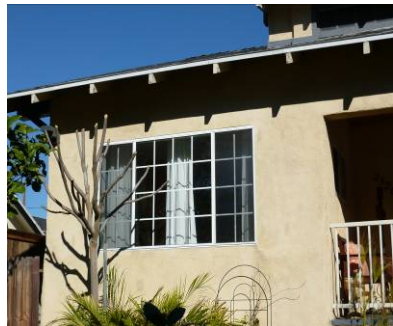
Not this: mullions were removed and flush window was installed instead of recessed
