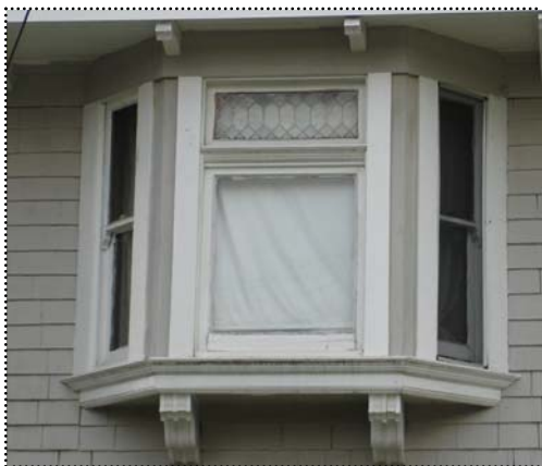
Below: This oriel window has characteristic component parts--wood double-hung sash as well as a stylized fixed upper sash in the center window.
