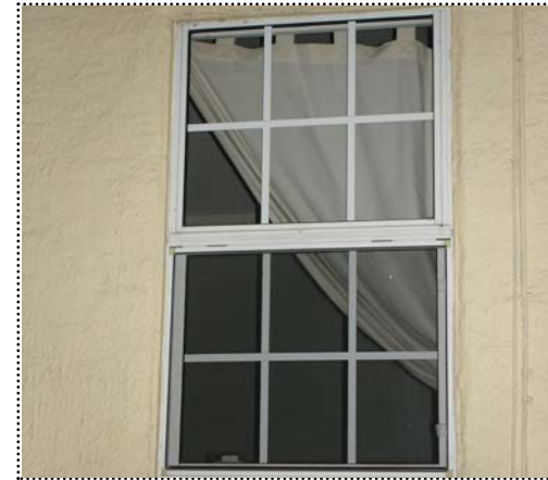
Above: This vinyl window has fake muntins or "grids," which are not appropriate for most historic styles.
