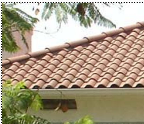
Below: Ridge caps of red tiles are a simple decorative feature that should be retained when roof work is undertaken.
