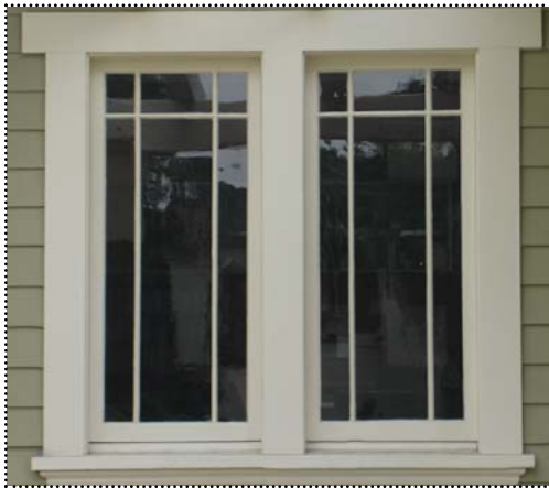
Above: Windows often have vertically oriented mullions with a cross muntin occurring only at the top of the window.
