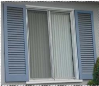
Below: This replacement aluminum sliding window does not give the same proportion to the facade as the original window.
