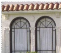
Below: These arched windows on a Spanish Colonial Revival house have decorative muntins and a red tile hood.
