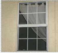
Above: This vinyl window has fake muntins or "grids," which are not appropriate for most historic styles.
