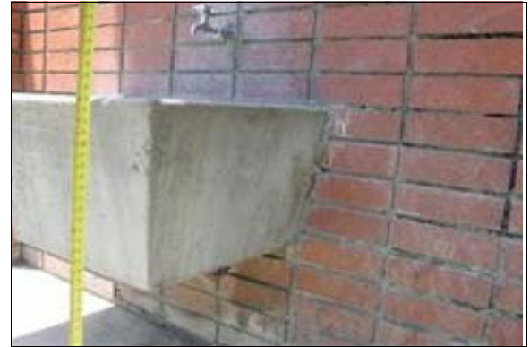
Sink at the Outdoor Dining Area
