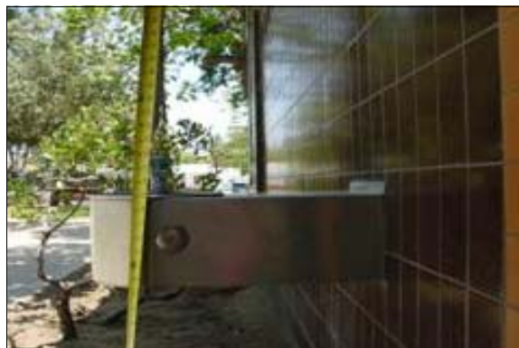
Drinking Fountain at the Restrooms
