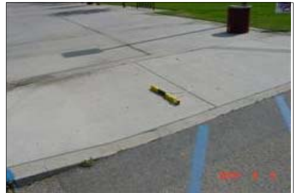
Curb Ramp at the Accessible Parking Spaces Outside of the Office (Right)
