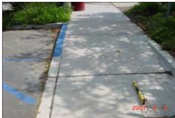
Curb Ramp at the Accessible Parking Spaces Next to the Baseball Field (Right)
