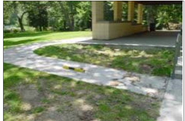
Path of Travel to the North Restrooms
